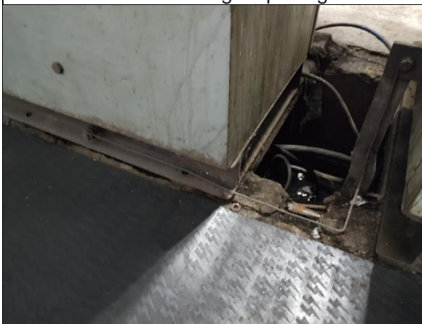
Water accumulation in Cable cellar
