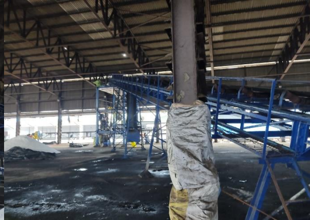
Conveyor belt for Bagging Machine
