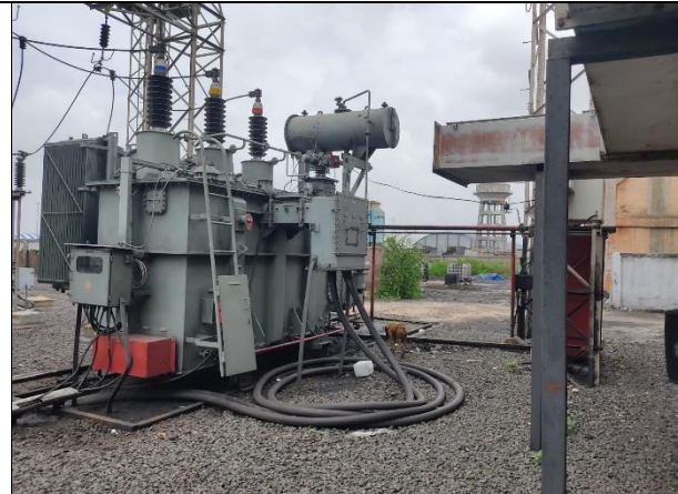
10 MVA transformer with NIFPS
