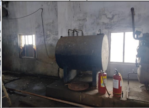
No curbing for diesel tank Oil Jetty pump room 2
