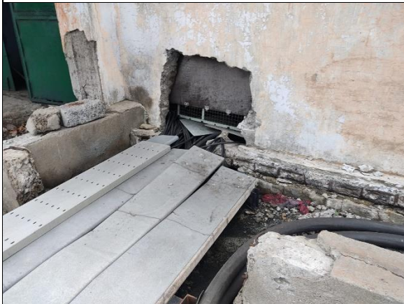
Cable Passage Opening
