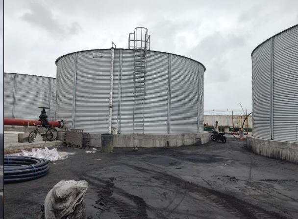
Dust Suppression System Water Tanks
