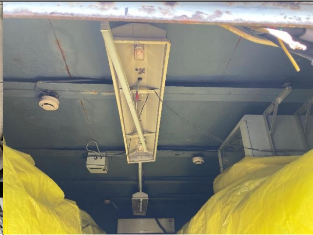
Smoke detectors at waft crane no. 5- not working
