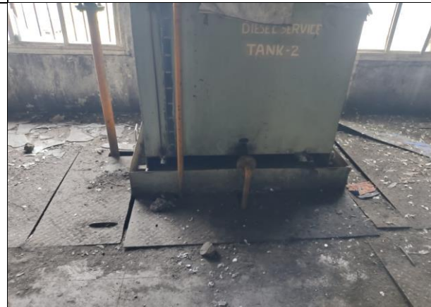
Inadequate curbing for diesel day tank
