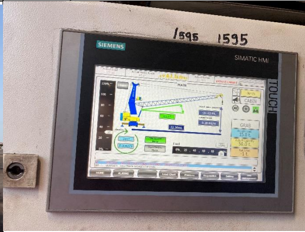
MHC Crane Panel at Operator Panel Room
