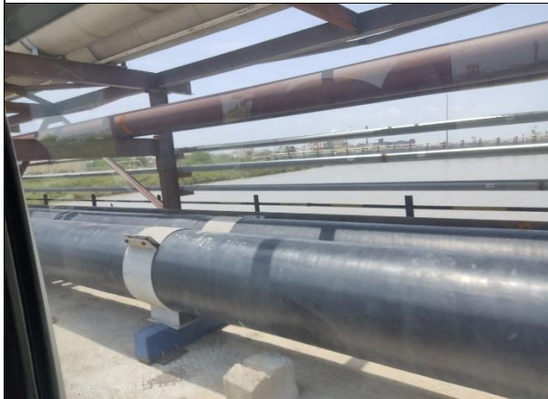
LPG Pipeline from Oil Jetty to IOCL
