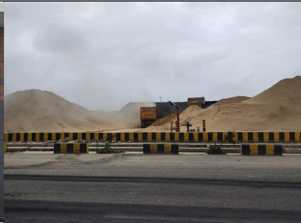
Dust Suppression Sprinkler at Sulphur Yard
