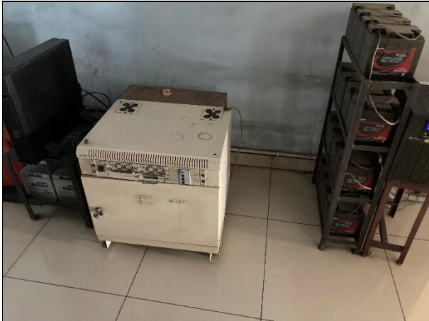
UPS and Battery Bank at Vehicle Traffic Management Building
