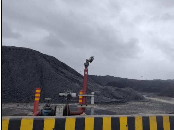
Dust Suppression Sprinkler at Coal Yard
