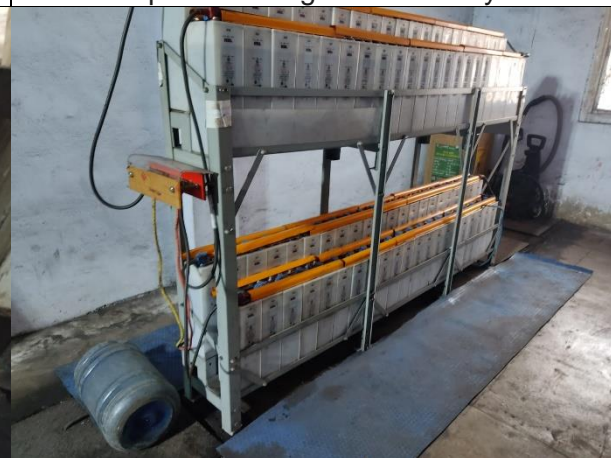
Battery Bank - Not Anchored to floor
