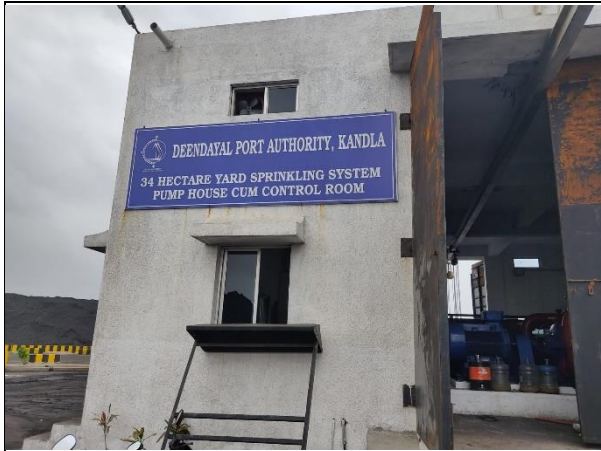
Dust Suppression System Pump Room 34 Ha
